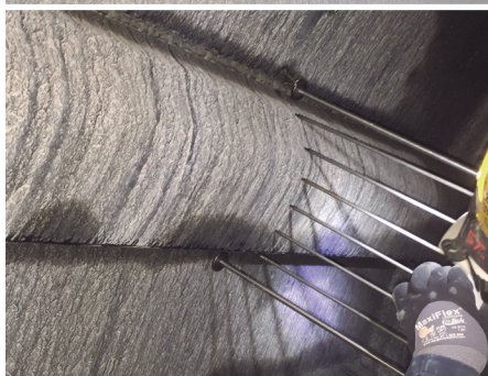
Top and Middle: Vulco® mill liner with R67 rubber compound installed in ball mill.
