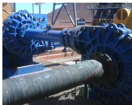
Warman® AHP slurry pump installation
