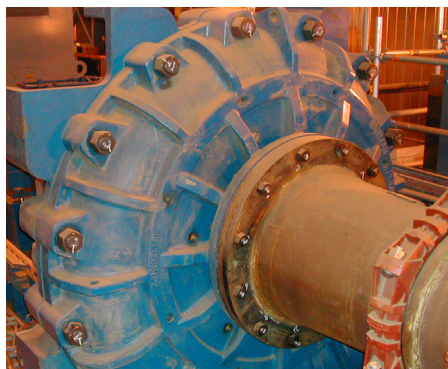
Warman® L slurry pump installation
