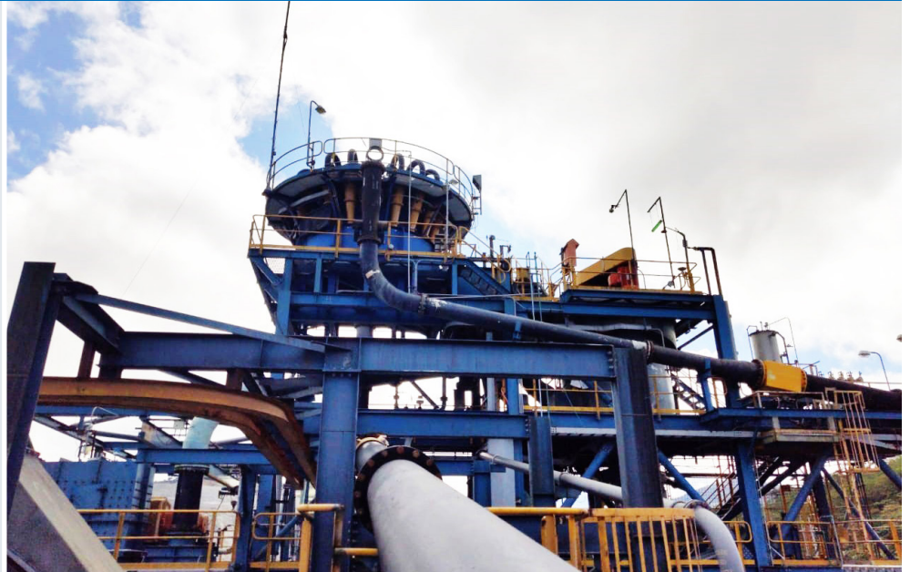
Right: Cavex® 400CVX10 hydrocyclone cluster on site
